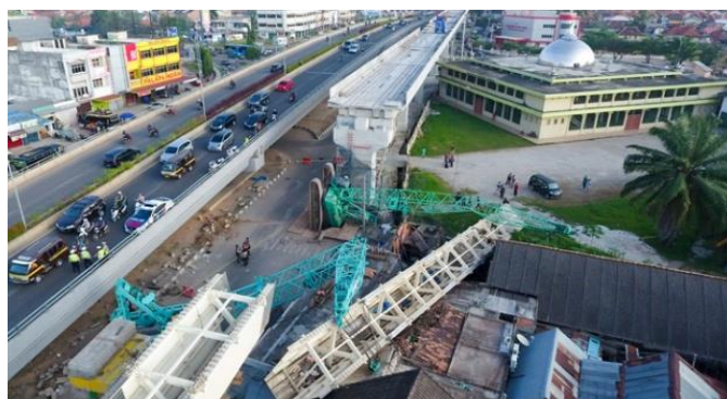
Figure 1. Condition of the Collapsed Crane
